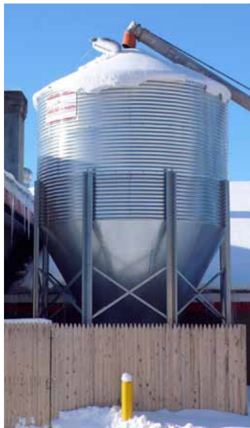
Left: Wood pellets delivered in bulk quantities are conveyed from the delivery truck into an onsite storage silo. Much of the infrastructure for conveying and storing wood pellets is identical to that used for grain in farming applications.
