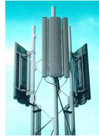
Courtesy Ericsson MW, Sweden
